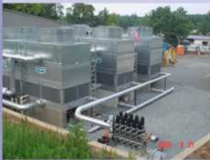
Turbo-Disc System installation on the GA College Cooling Tower
