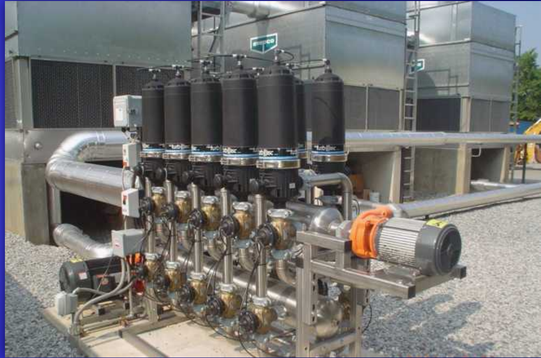
800-GPM Turbo-Disc Side-Stream Skid System
