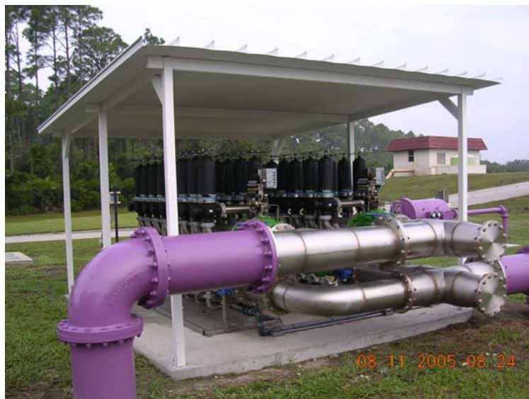
Custom Type 316 stainless steel manifolding fabricated by Miller-Leaman to accommodate future expansion of the Turbo-Disc Filter system
