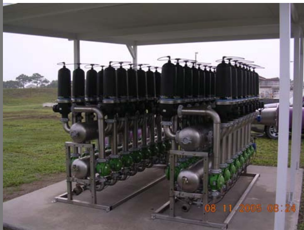
Miller-Leaman’s automatic Turbo-Disc Filter system installed at Dunes Utilities; current filtration capacity is approximately 4,500 GPM
