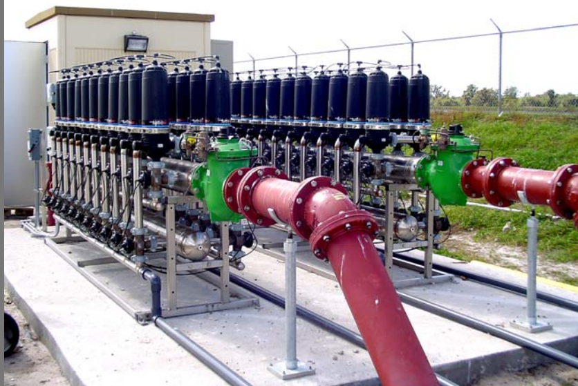
Outlet Water Piping from Miller-Leaman’s 1,400 GPM Turbo-Disc Filtration System
