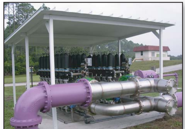
Dunes Utilities – Reclaimed Water Filter Station. Filtering Reclaimed Water used for Irrigation.
