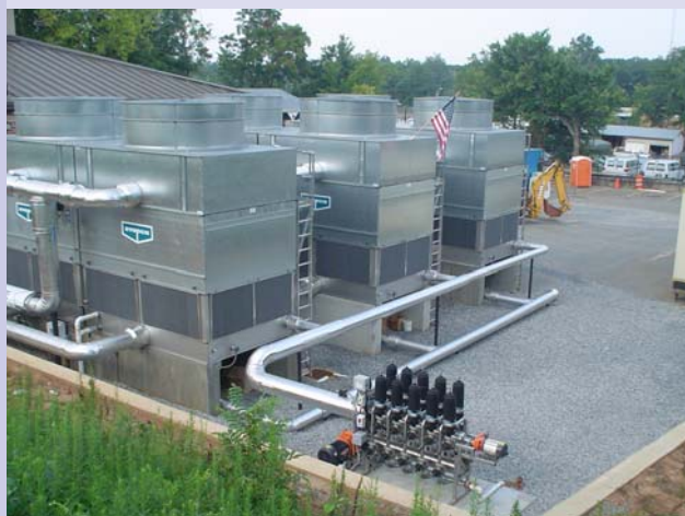
Turbo-Disc System Installation on the GA College Cooling Tower
