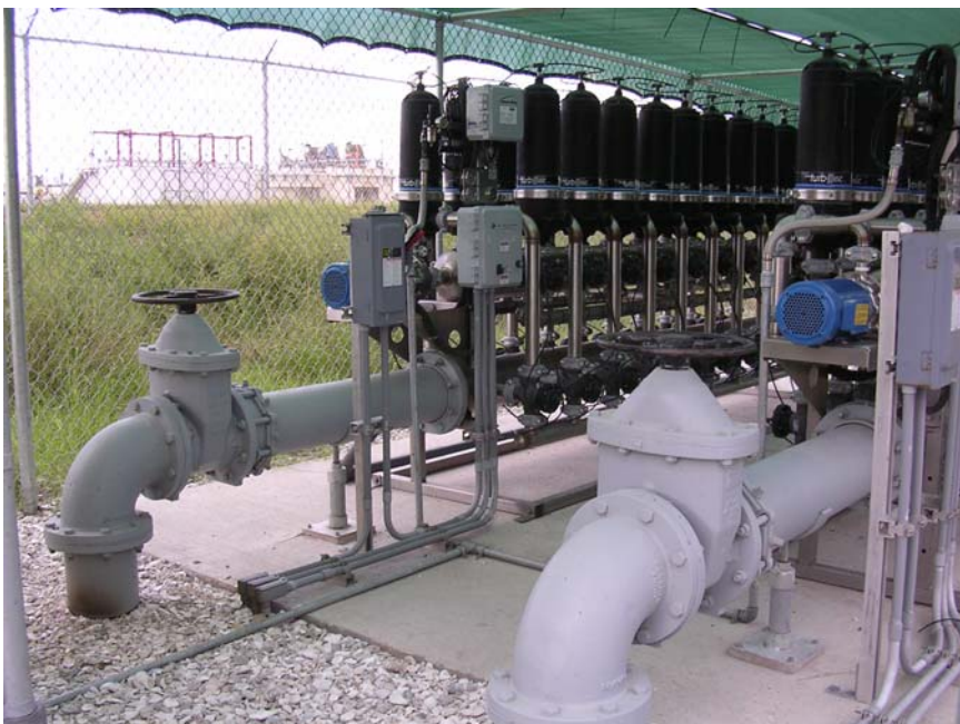
Intake Water Piping to Turbo-Disc System with Booster Pumps
